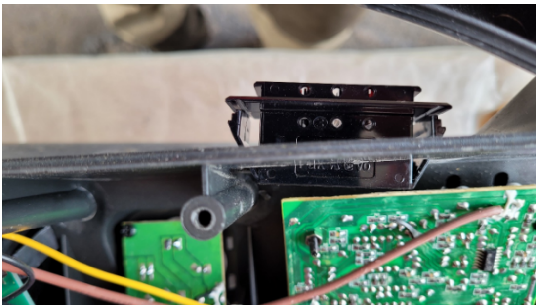
Photo 16 - tight clearance inside the box for the PowerPole outlet.
