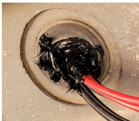
Photos 8 and 9: The power and coax cables drop out of the engine compartment and run alongside the chassis to reach the through hole grommet at the passenger footwell.
