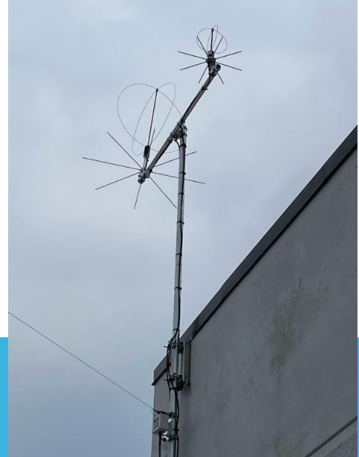
Backup Satellite Antenna System
