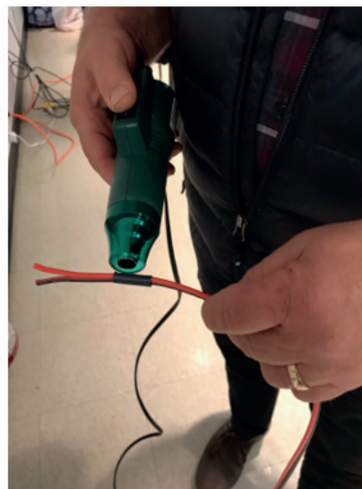
Heat Shrink Tubing being Shrunk
