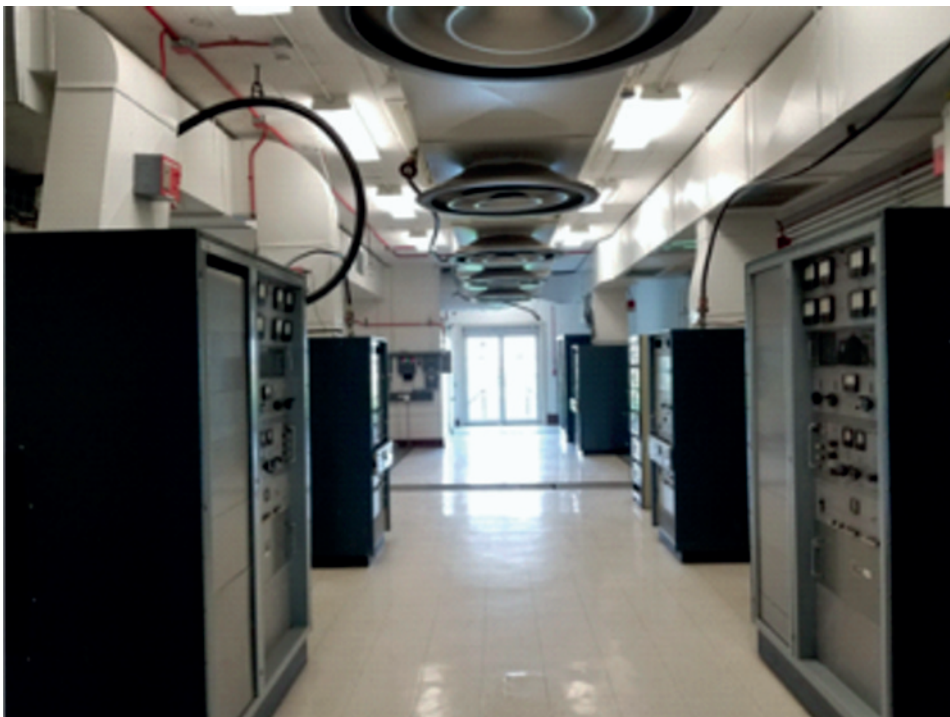
Corridor of 3 CHU Transmitters on 3.33, 7.85 and 14.67 MHZ inside U99 building.
